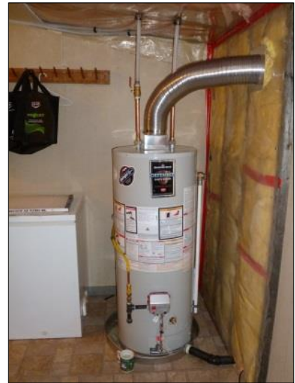
Figure 41 Direct vent propane HWH
