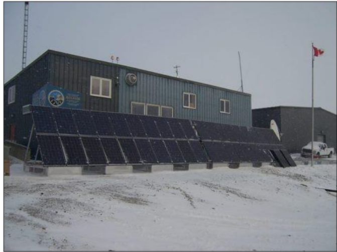
Figure 22 Installed Sachs Harbour PV system
