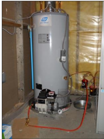
Figure 42 Oil-fired hot water heater
