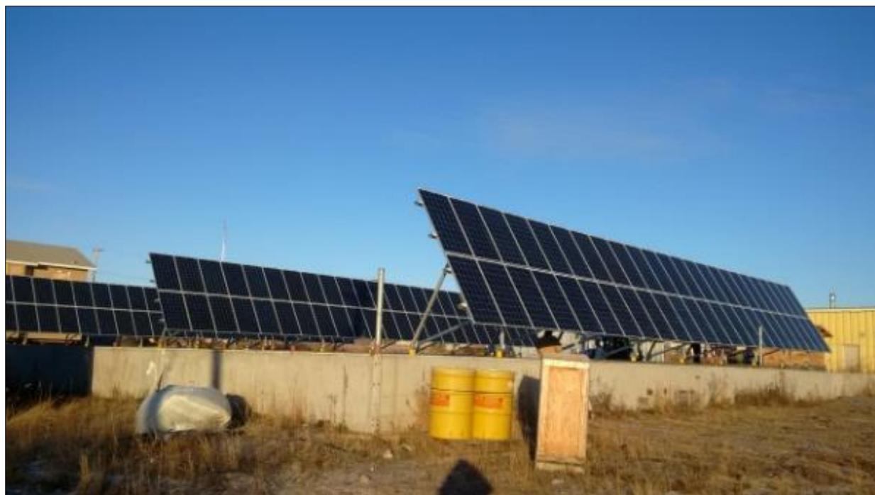
Figure 46 Lutsel K'e's Solar PV System Installed.
