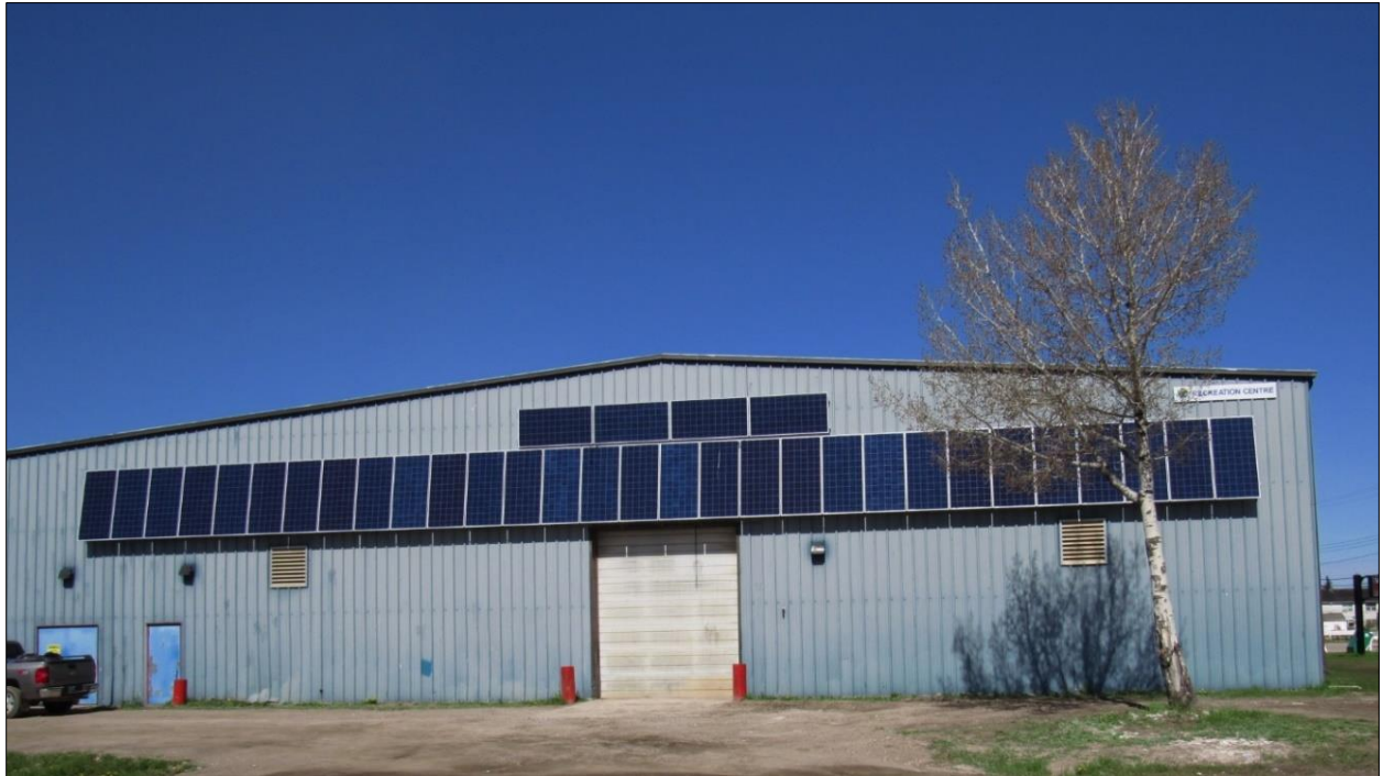
Figure 40 Fort Simpson Arena, wall mount solar system
