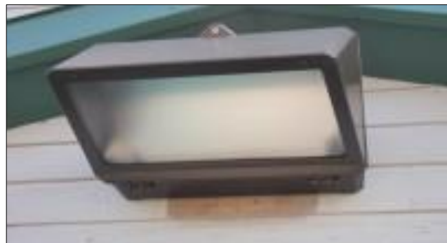
Figure 15 Exterior LED Lighting Wekweeti
