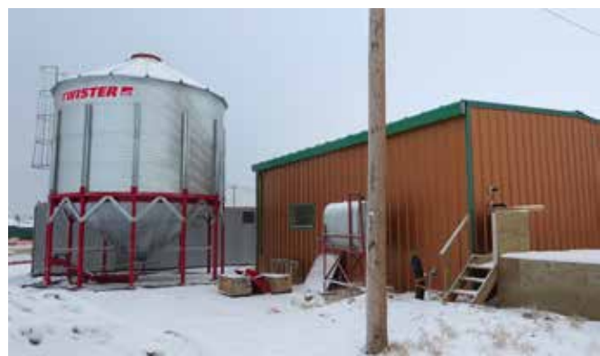
The pellet hopper for the district heating system, with the boiler container in the background.
