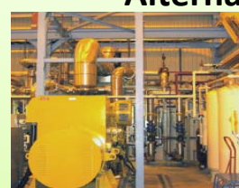
Waste Heat Recovery
