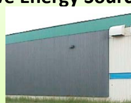
Solar Air Heating
