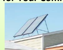
Solar Water Heating
