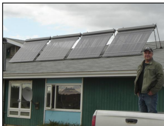
Figure 1 – SWH Tubes at Fort Providence
