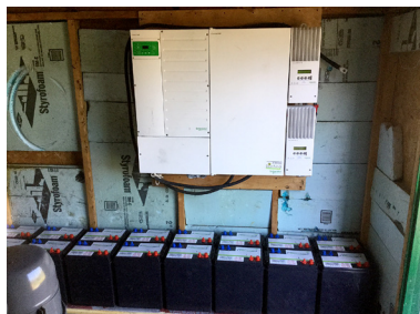
The batteries and inverter that provide useful power to the camp.
