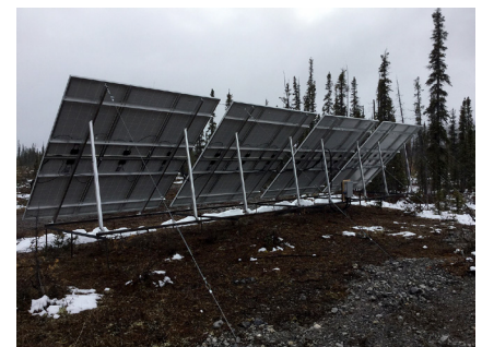
Ground-mounted racking of the solar panels at a 45-degree angle.
