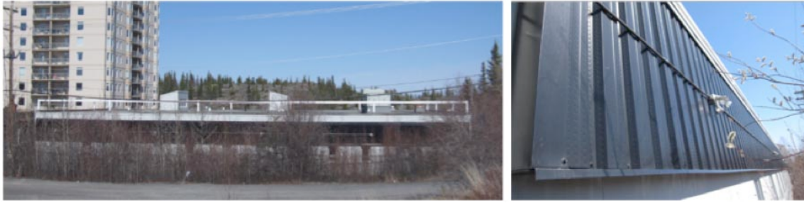
Figure 3. SolarWall at the GeoScience Building, Yellowknife
