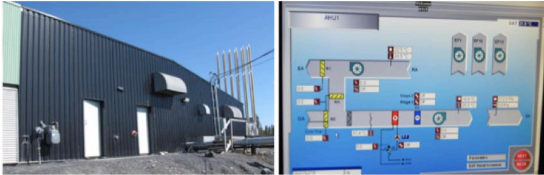
Figure 6. Left: SolarWall at Female Young Offenders Correctional Facility, Inuvik; Right: Honeywell Building Control System Interface showing SolarWall controls
