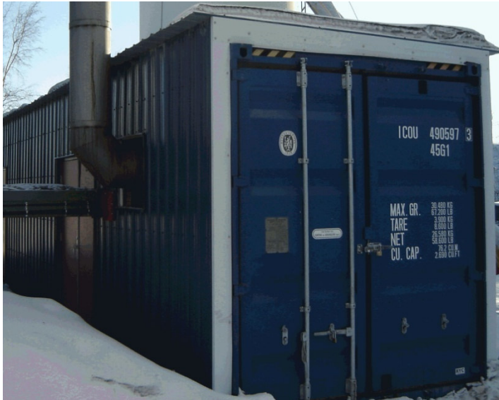
Photo: AEA. Northern Property REIT boiler system enclosed in a siding clad intermodal container at Garden Apartments in Yellowknife.
