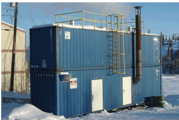
Photo: AEA. NPREIT Pellet boiler system at Bison Apartments using a stacked intermodal container as storage.
