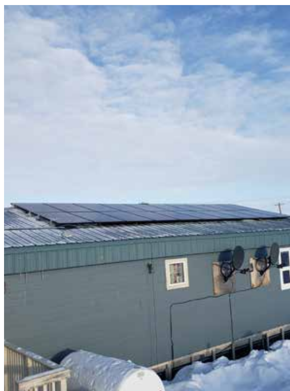
Solar panels on a building in Paulatuk.
