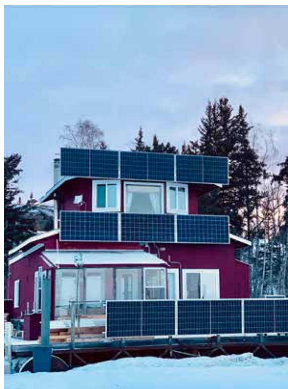
Solar panels on a houseboat in Yellowknife.
