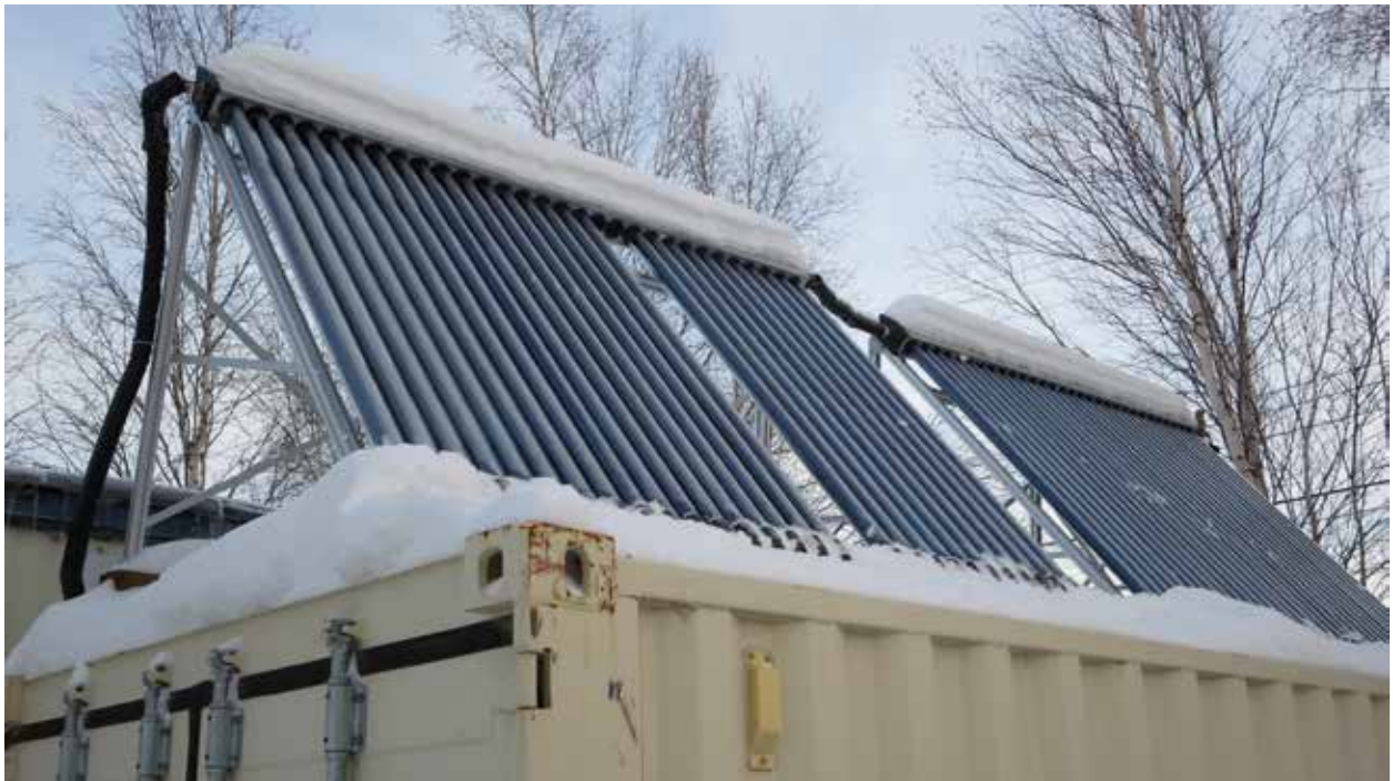
A new solar hot water system in Norman Wells, which received a rebate under our Alternative Energy Technologies Program.
