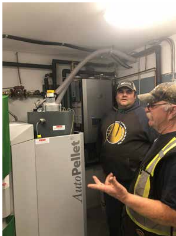
Norm Prevost from Prevost Electric Ltd. (right) talking to Derek, our Dehcho Regional Energy Project Coordinator (left) about the wood pellet boiler in the Kát'odeeche First Nation's new youth centre. The highly energy-efficient building also boasts a 10.5 kW solar system.
