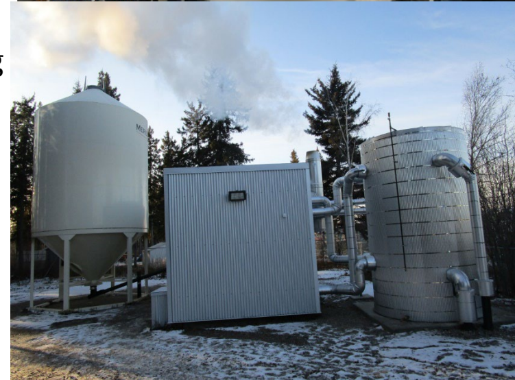
(Hay River Schools District Plant – Thermal Storage)
