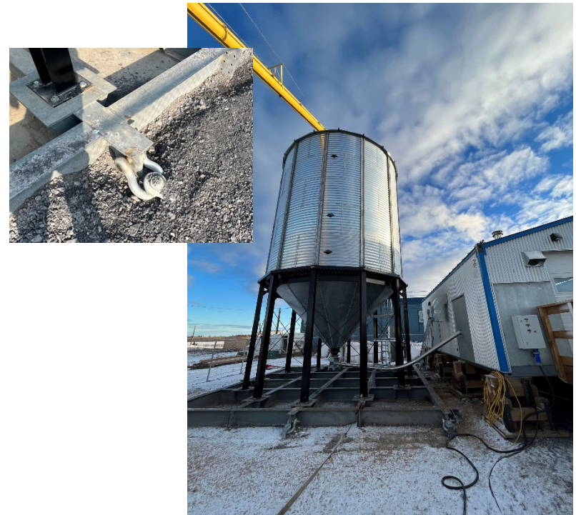
(Aklavik School Biomass Silo/Foundation)
