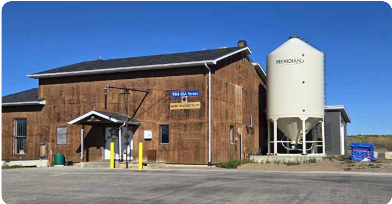
The large, white silo is a telltale sign of the new wood pellet boiler at the water treatment plant in Fort Simpson. This year, the Village of Fort Simpson won the Canadian Biomass Project of the Year award for their efforts in switching their community buildings over to biomass heating.
