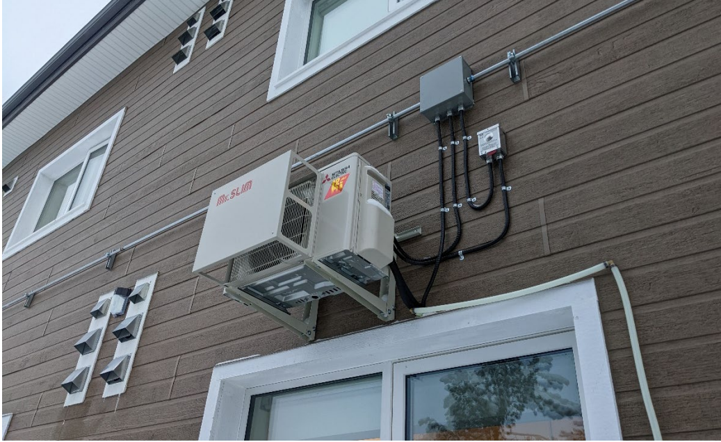
One of the outdoor heat pump units.
