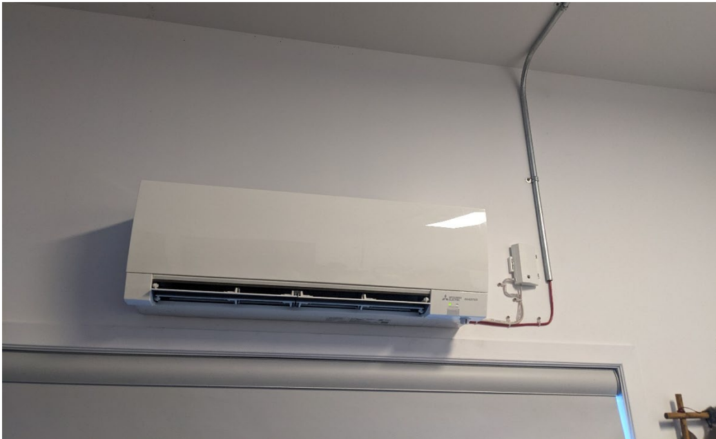
An indoor head unit for the heat pump.
