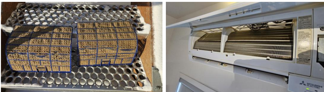
Figure 3.7 – Dirty filter from Unit A (left) and missing filter in Unit C (right) as observed in November 2024.
